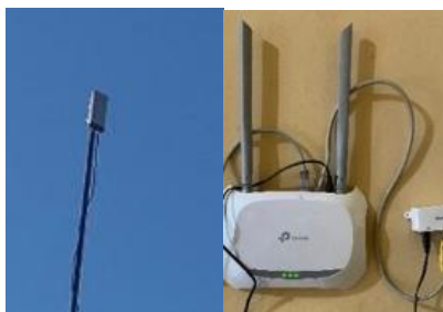
Gambar 5. Pemasangan Router Penerima (receiver) ke router TP-Link
